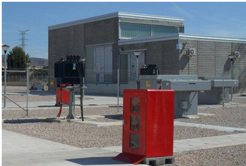
Figure 33 Substation of Crevillente.
