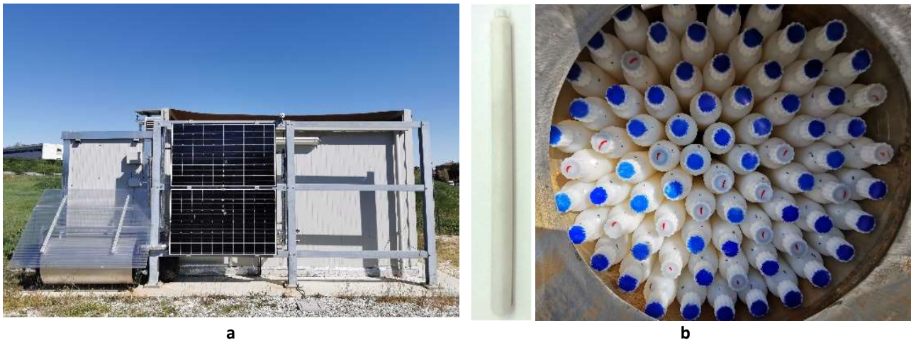
Figure 3-24: PV/T panels installed on the south facade of the mock-up with the PCM-tank on the left (a); detail of TubeICE S10 (marked in blue) and S32 (marked in red) filling the storage tank (b).
