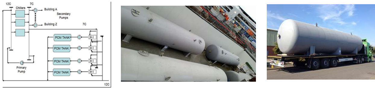
Figure 3-9: Installed TES capacity 4 \times 60 \text{ m}^3 +13°C PCM solution providing total 10,000 kWh [5].
