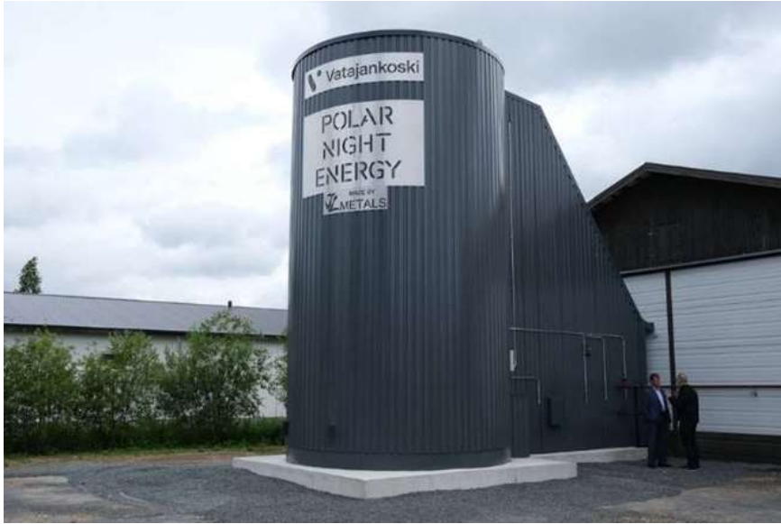
Figure 4-11: Sand-based STES installation in Finland [22].
